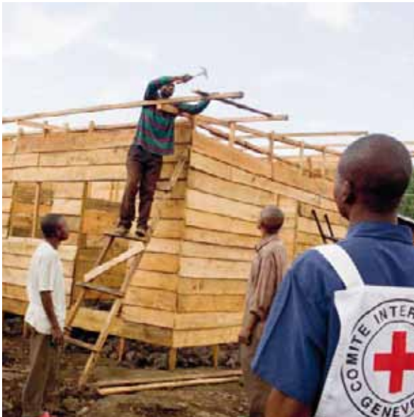
Construction of the Covedec Center for orphans or children separated from their parents in Goma, Democratic Republic of Congo. The center is run by Pastor Patrick Sengoza, who currently cares for around 130 orphans with the support of the ICRC.
